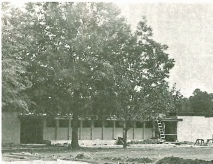
HOLIDAY MOVE —With the move scheduled for the Christmas holidays, the new Engineering, Mathematics and Physics Building will be ready for use next semester. Mechanical drawing, math, and physics courses will be conducted in the well-equipped building. (Photo by John Sullivan)
